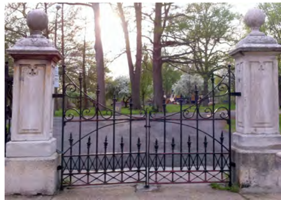
One of the park entrance gates in need of repair.
